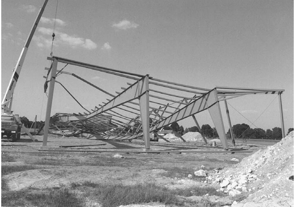
FIGURE 16.5 Pre-engineered building collapsed during erection. (Photo: Prof. Duane S. Ellifritt.)
